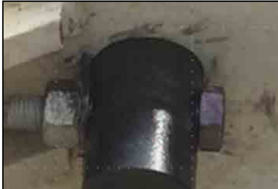
Corroded support pins.
